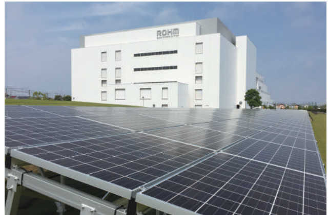
Solar panels at ROHM Hamamatsu
